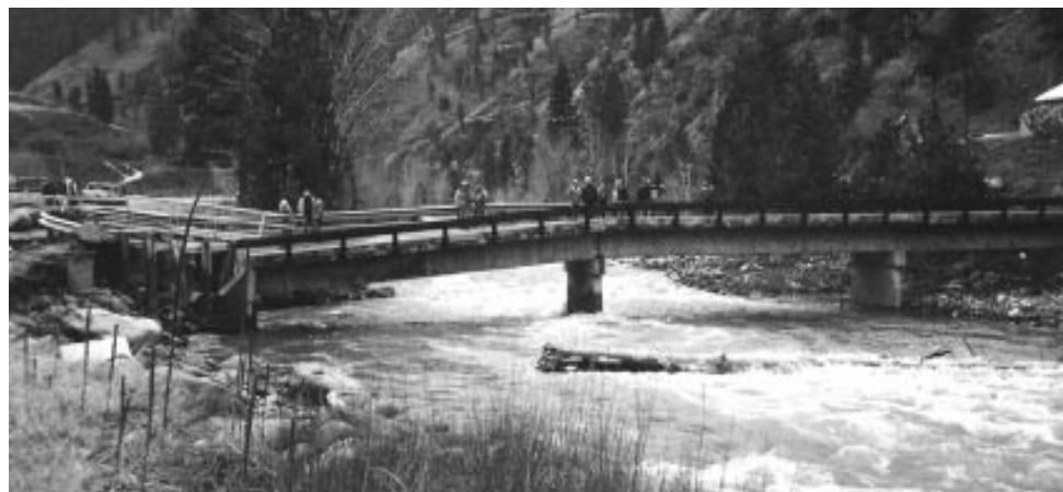
Figure 1.1 Little Salmon River Bridge, Nez Perce National Forest. A January 1997 flood event scoured the abutment and one of the intermediate piers causing failure (Kattell & Eriksson,1998)
