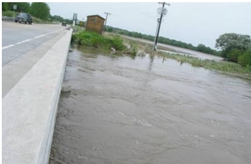
Figure 2.3 Photo. Partially inundated bridge deck at Salt Creek, NE
